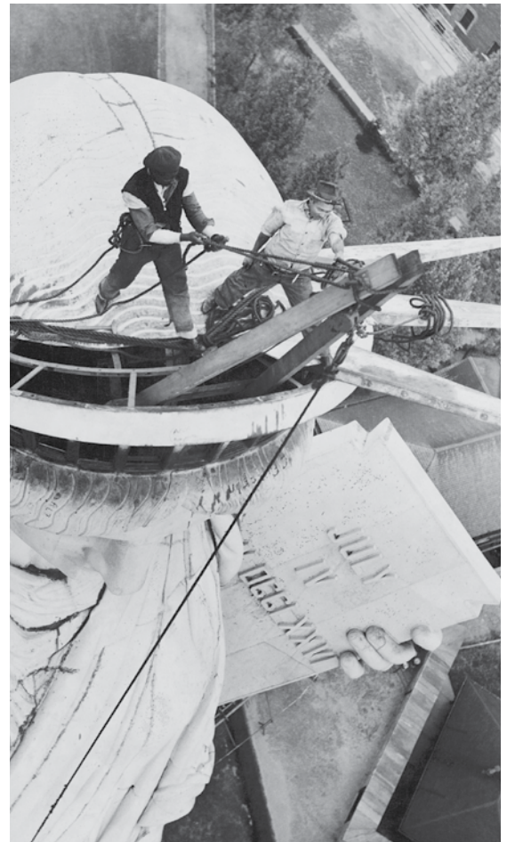
Renovation Work on Statue of Liberty. This picture was taken from the torch which she holds. Sept 26th 1938. © Hulton-Deutsch Collection/CORBIS
